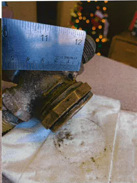
Measurement of pinhole leak
